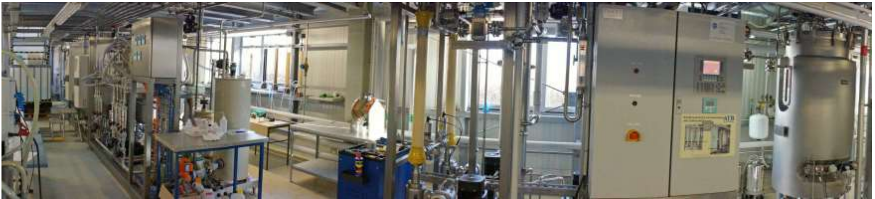
Pilot plant facility for lactic acid fermentation at Leibniz Institute for Agricultural Engineering and Bioeconomy (ATB Potsdam)
